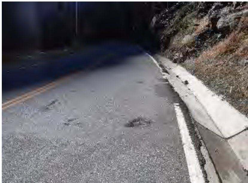
Figura 6: Baches peladuras carretera central Km 87+620
